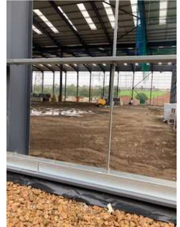
View from rear of building, through building with front elevation in background
